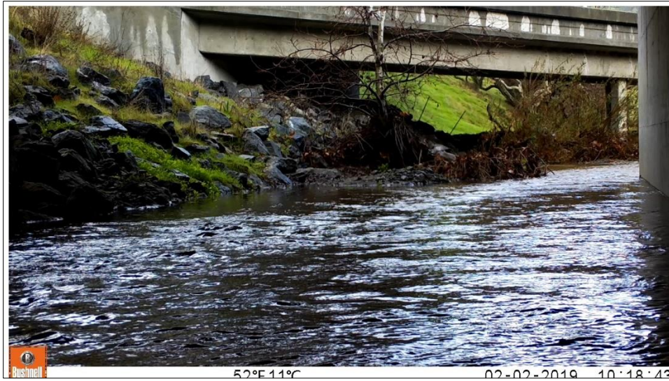
Figure 16. Cedar Creek bridge flooded during February 2019.
