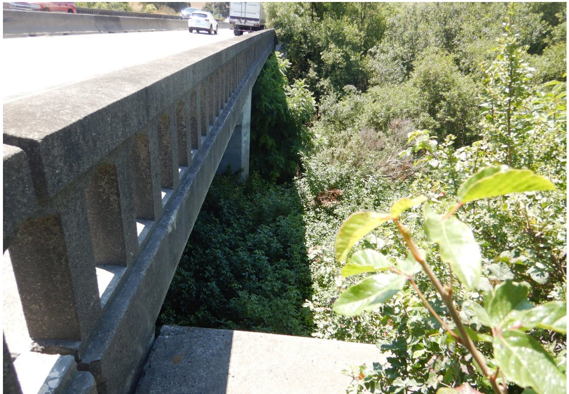
US 101 Site 5 Pajaro River Bridge. Photo taken from north side Pajaro River on west side of US 101 southbound looking south.
