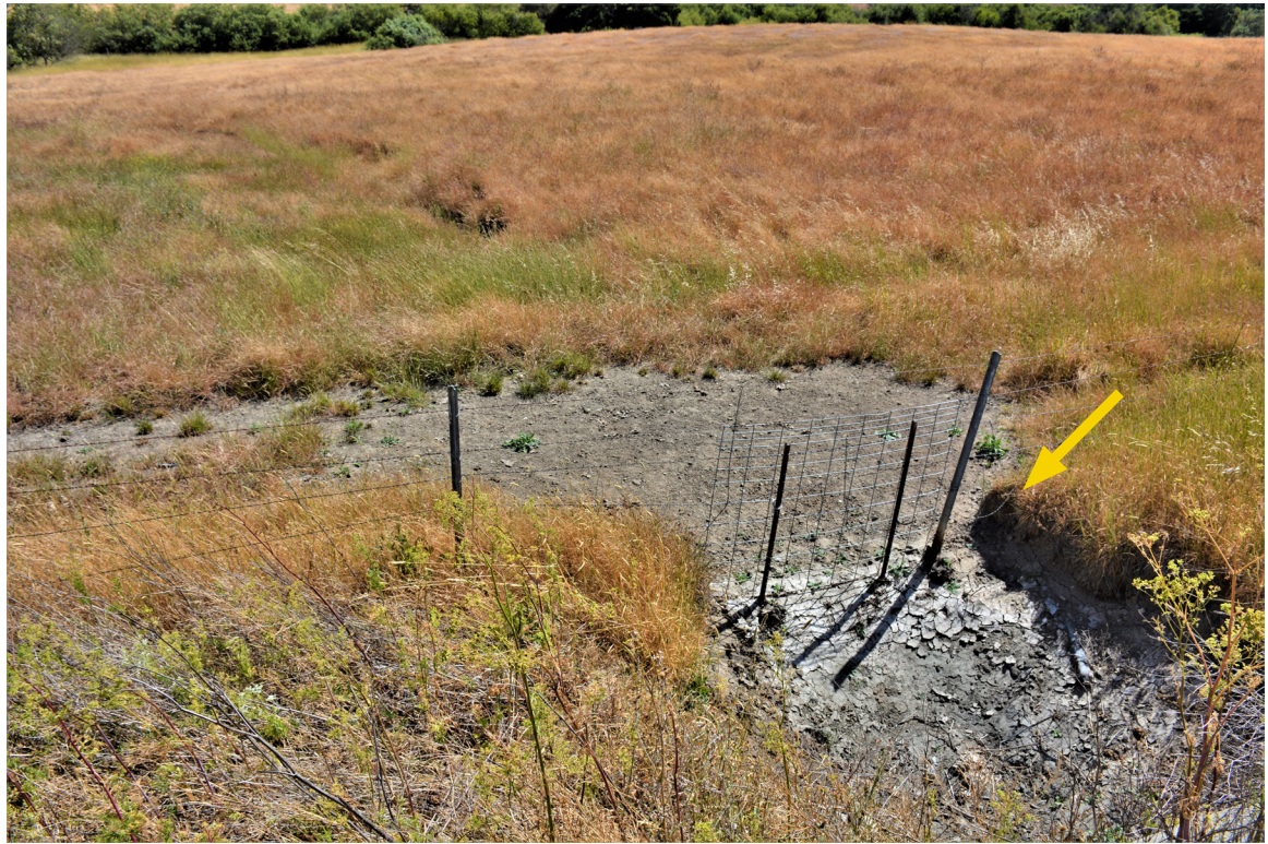
SR 156 Site 4. View of fence and section of loose barbed wire strands. Loose barbed wire strands are indicated by yellow arrow. Photo faces southwest.
