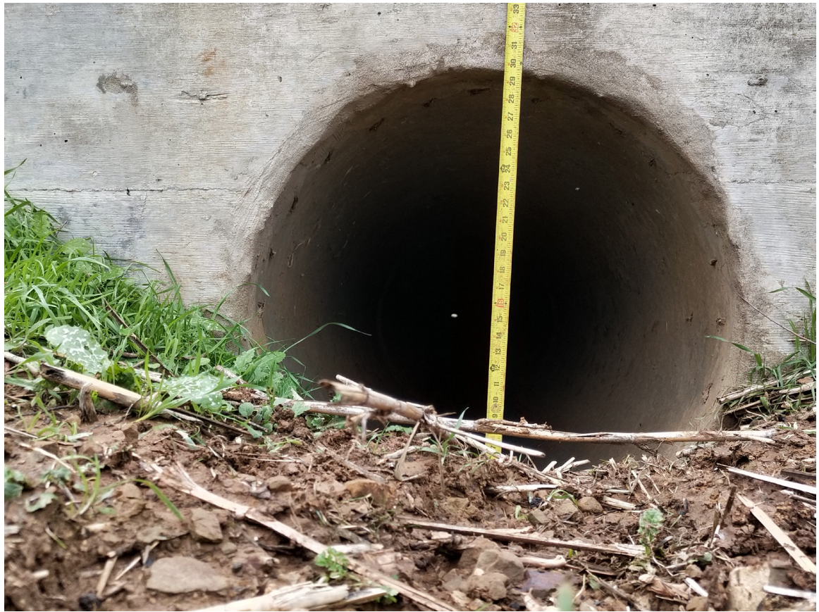
SR 152 Site 5 Coyote Puppy culvert. Photo of culvert entrance on SR 152 westbound side.
