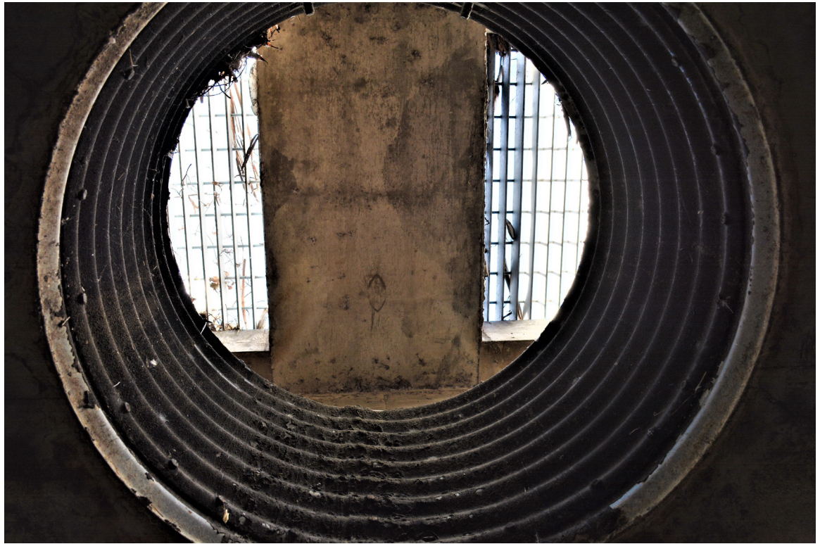
SR 156 Site 1. Circular opening in ceiling within middle of culvert with grate, median, then grate visible.
