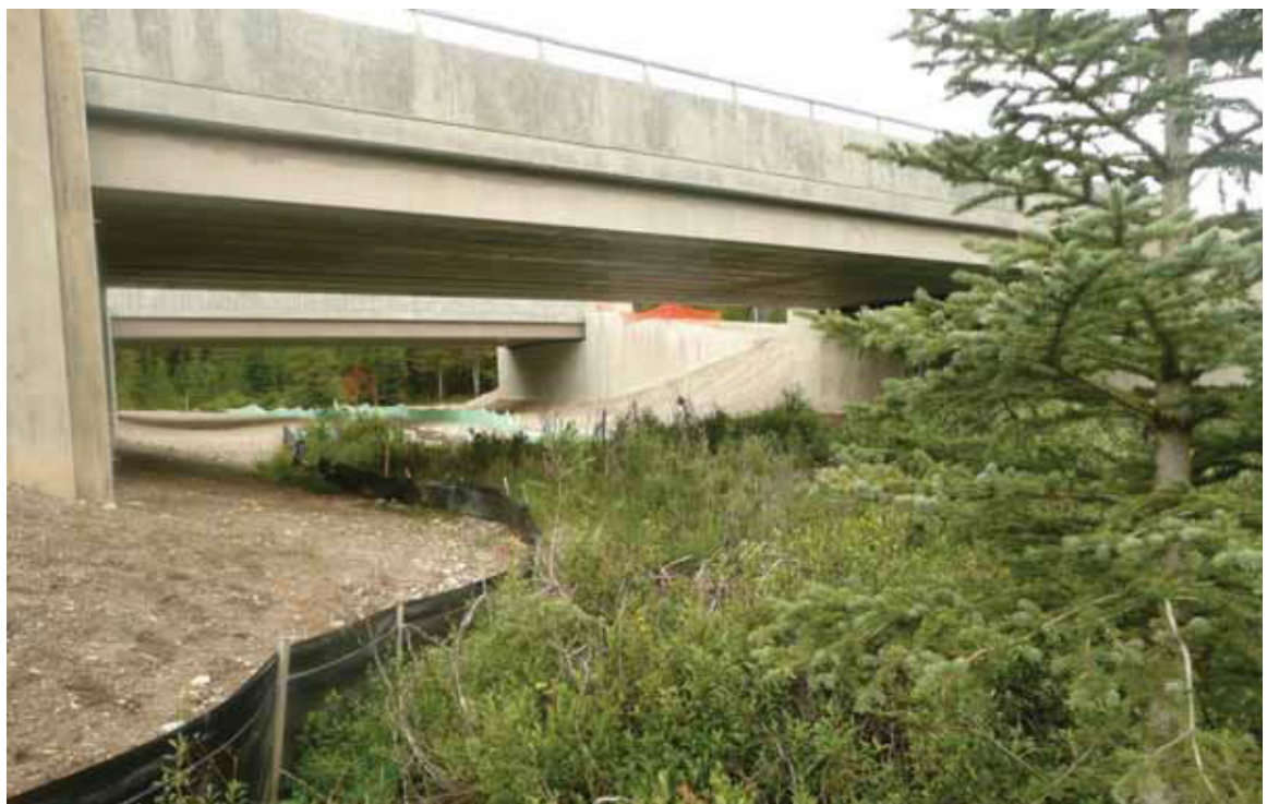
Example of a wildlife undercrossing designed to accommodate water flow. Photo by Tony Clevenger.
