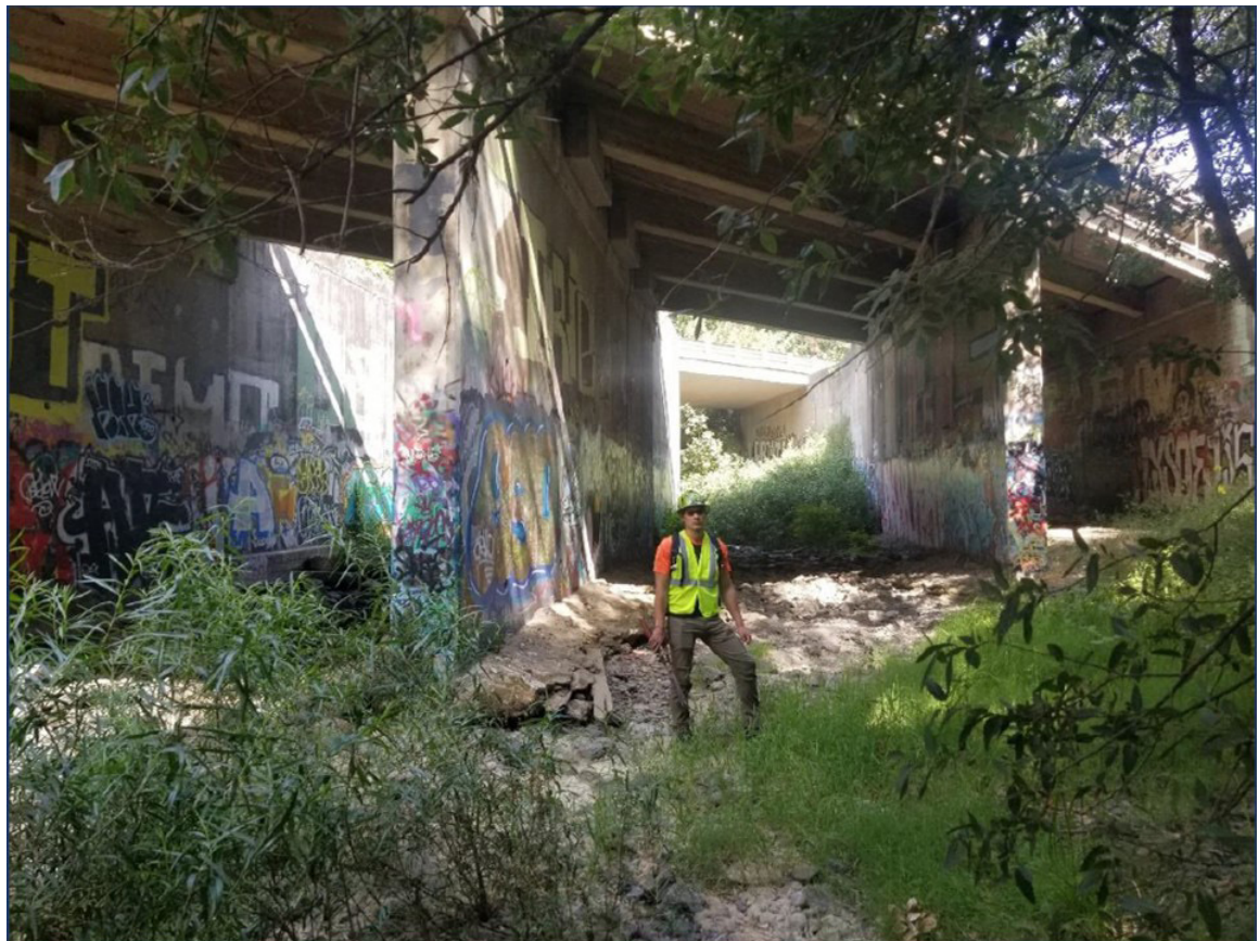
US 101 Site 1 Carnadero Creek Bridge. Photo faces northwest from the east side of the bridge.
