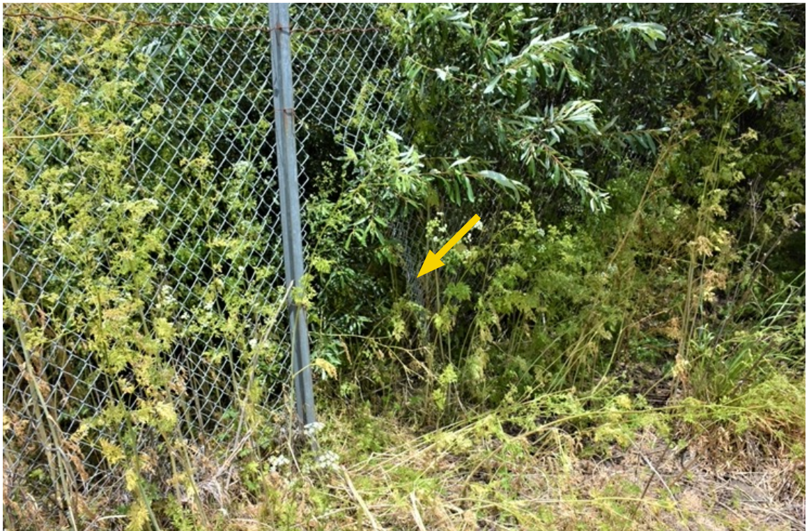
US 101 Site 7. Hole in the fence to the north indicated by yellow arrow.
