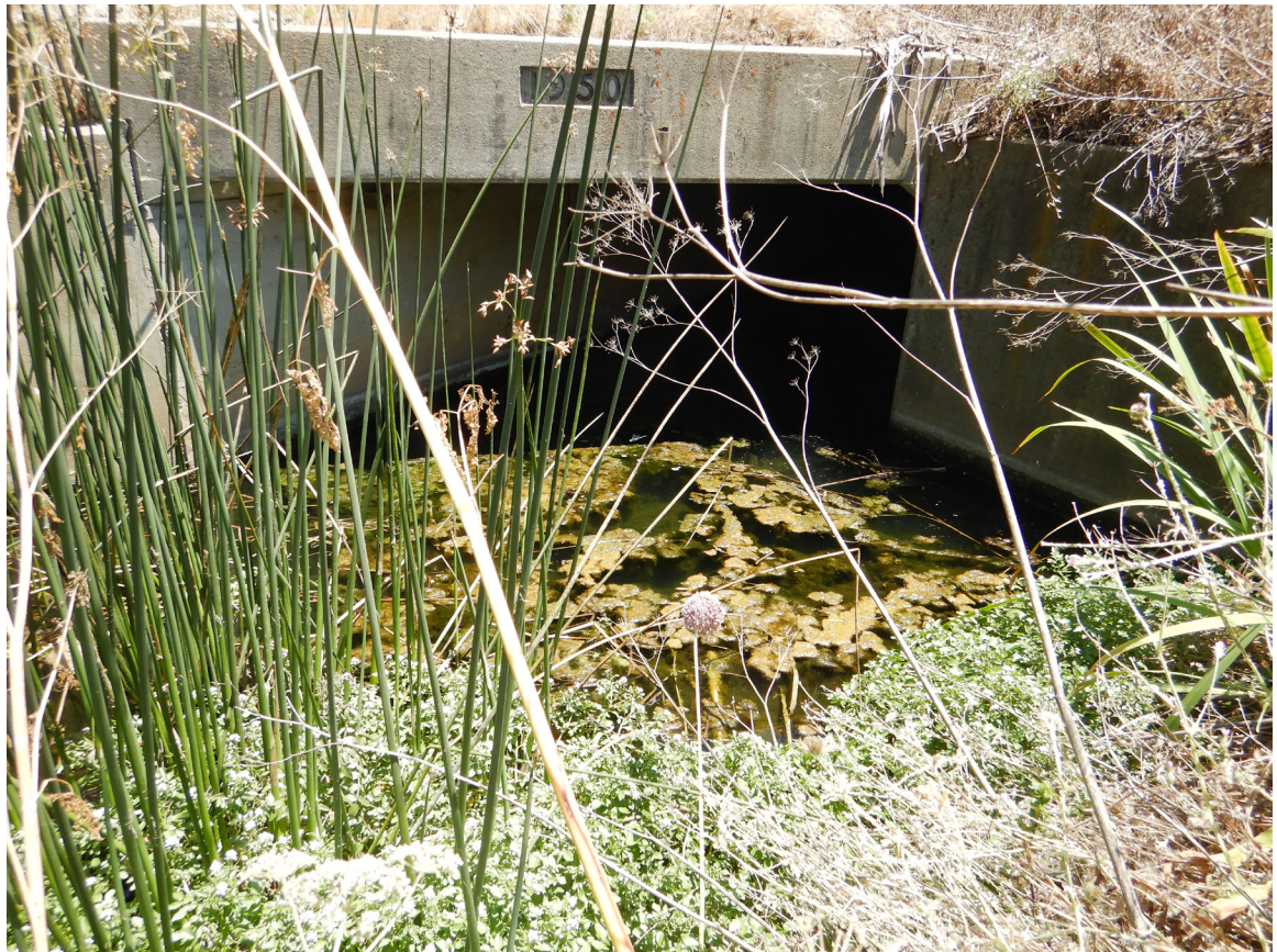
US 101 Site 2 Gavilan Creek culvert. Photo faces southeast towards the culvert entrance on the southbound side of US 101.
