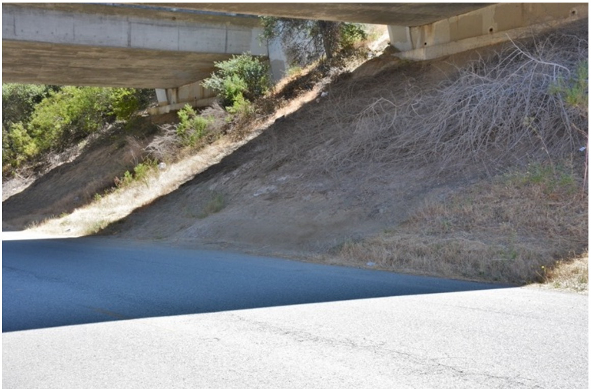
US 101 Site 4 Anzar Road underpass. Southern slope of shoulder leading up to US 101 overpass.
