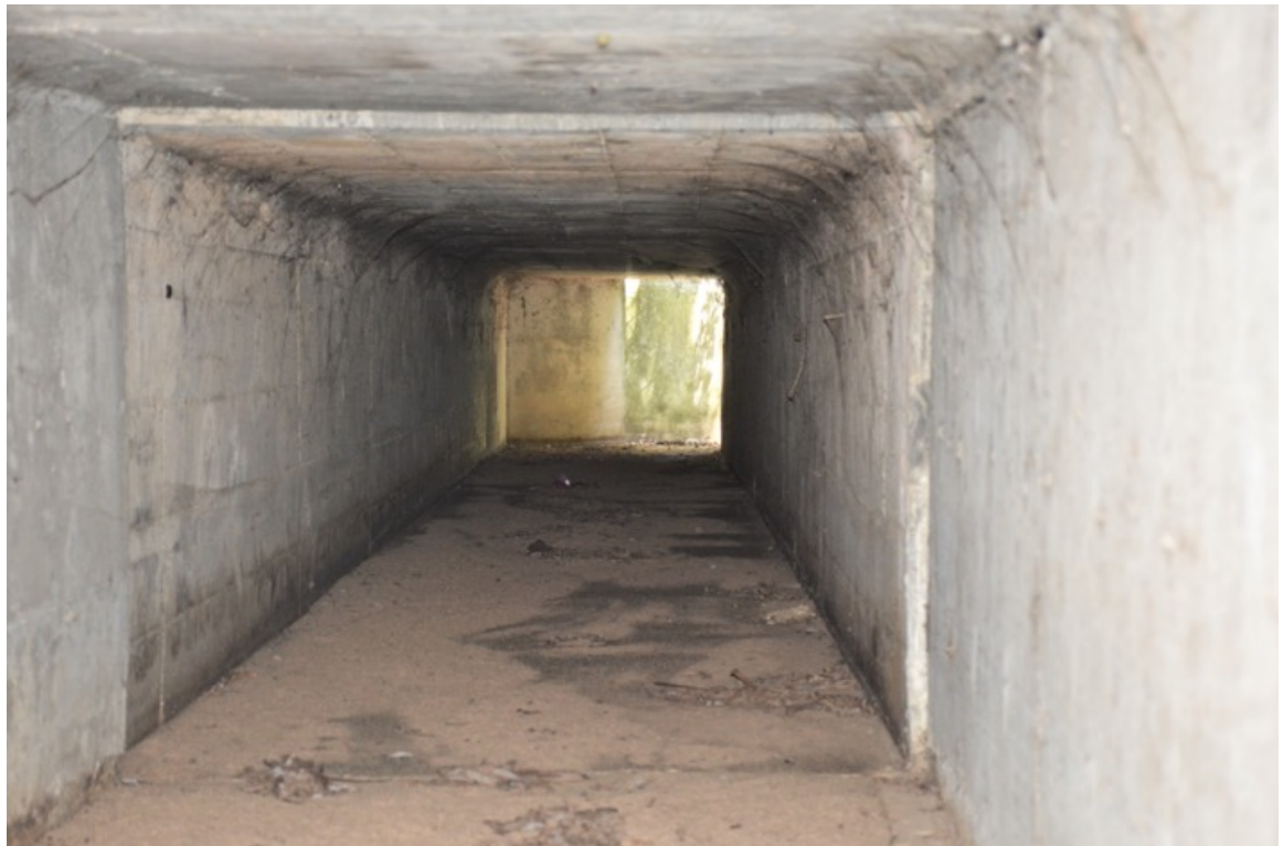
US 101 Site 17. Example from within western section of angle at southern opening. Photo faces south.
