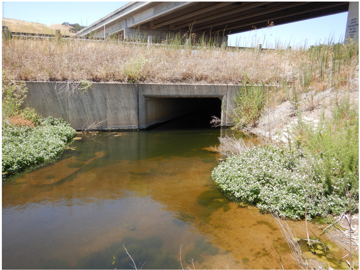
US 101 Site 2 Gavilan Creek culvert. Photo faces northwest towards the culvert entrance on the northbound side of US 101.
