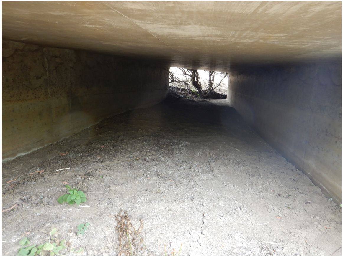
SR 152 Site 3 Ortega Creek Bridge. Photo from the SR 152 eastbound side of the bridge facing northeast.
