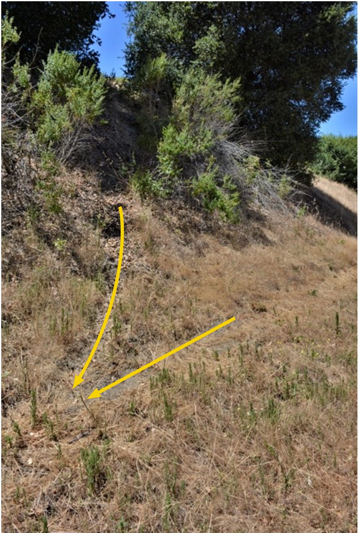
US 101 Site 4 Anzar Road underpass. Example of trails west of the southern shoulder. The yellow arrows highlight the trails and point to where the trails meet.
