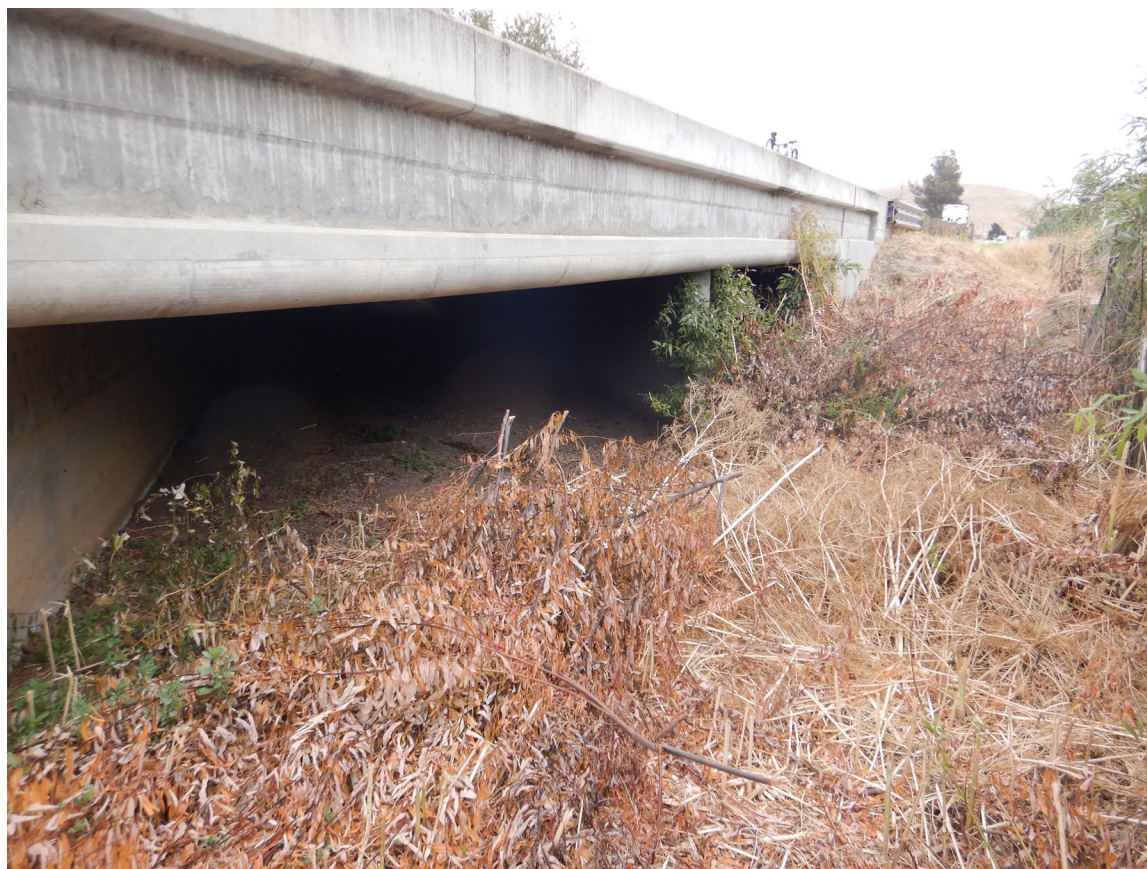
SR 152 Site 3 Ortega Creek Bridge. Photo taken from the SR 152 eastbound side of the bridge facing northeast.
