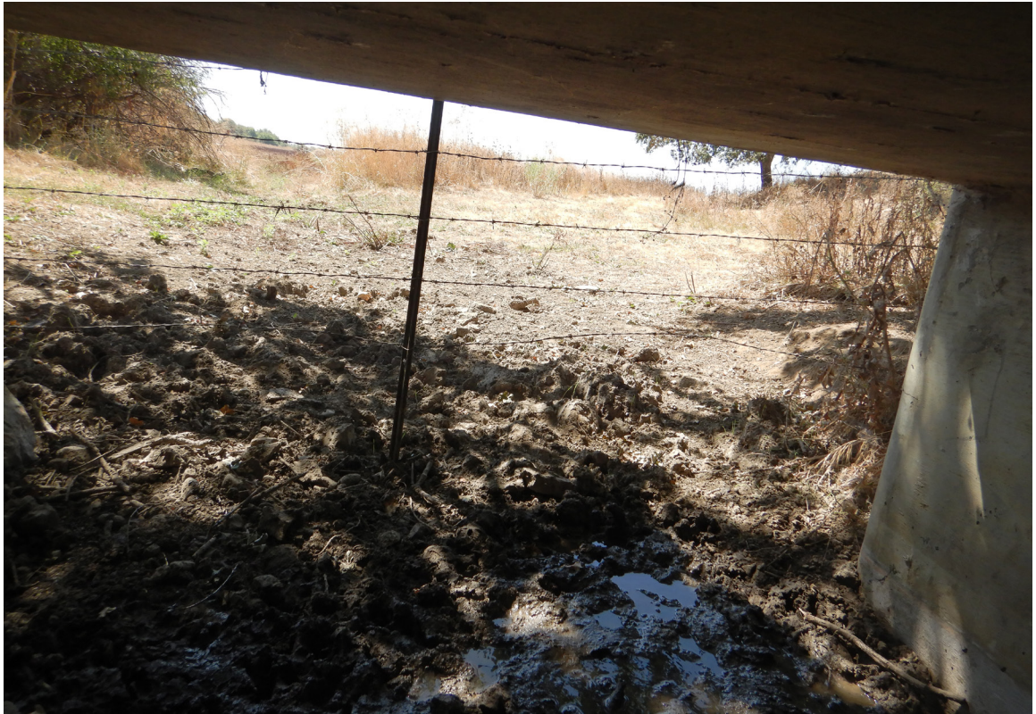
SR 152 Site 2 San Felipe Lake box culvert. Photo faces southeast away from the culvert entrance on the SR 152 eastbound side.
