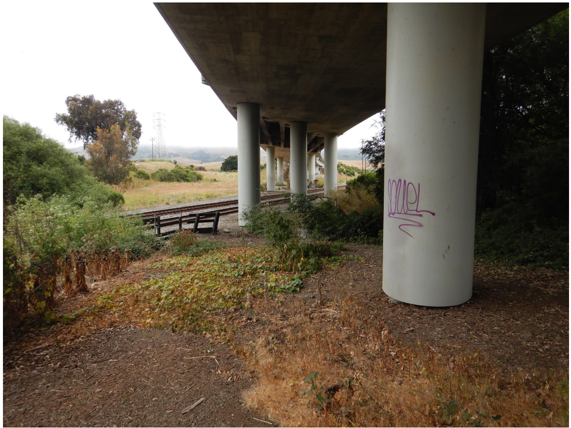
US 101 Site 4 Tar Creek overpass. Photo faces south/southwest from under northbound US 101.
