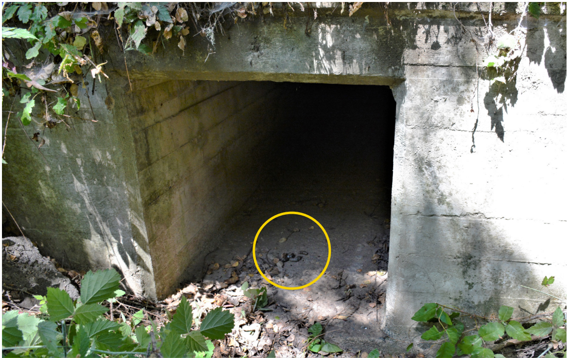
SR 129 Site 3. Close-up of southwest opening. Bobcat scat ( Lynx rufus ) visible in entrance of culvert (circled in yellow).
