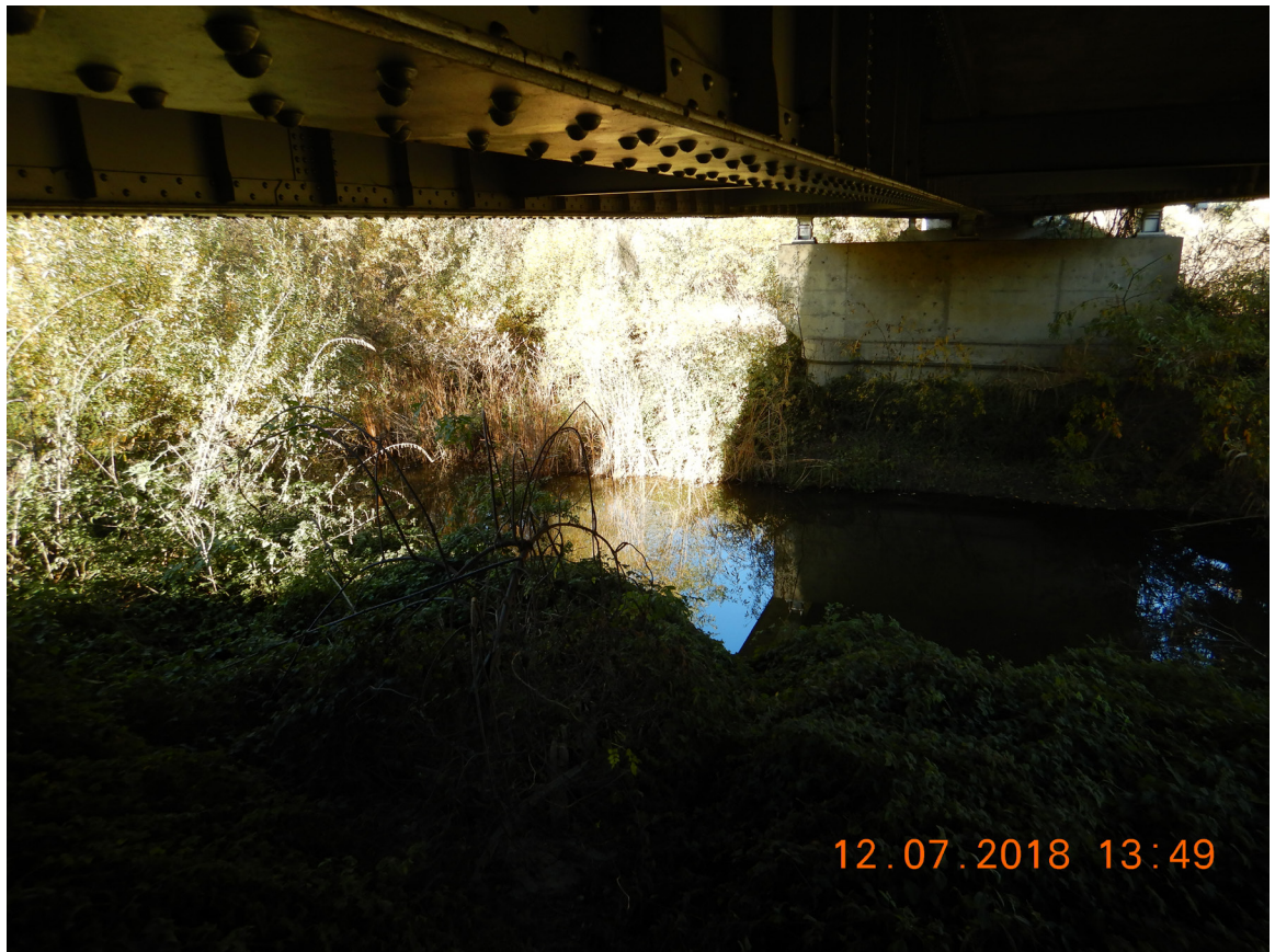
US 101 Site 6 San Benito River Bridge. Photo faces south taken from north side of San Benito River under US 101 northbound.
