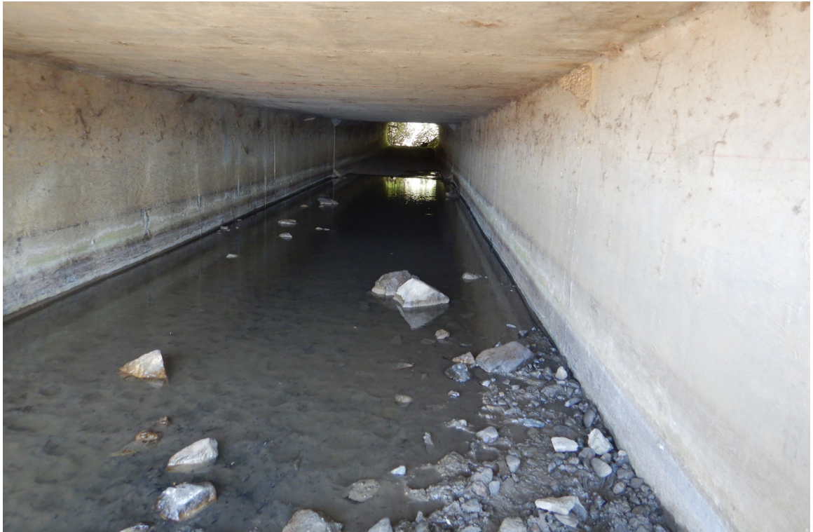
SR 152 Site 2 San Felipe Lake box culvert. Photo faces northwest through the culvert from the SR 152 eastbound side.
