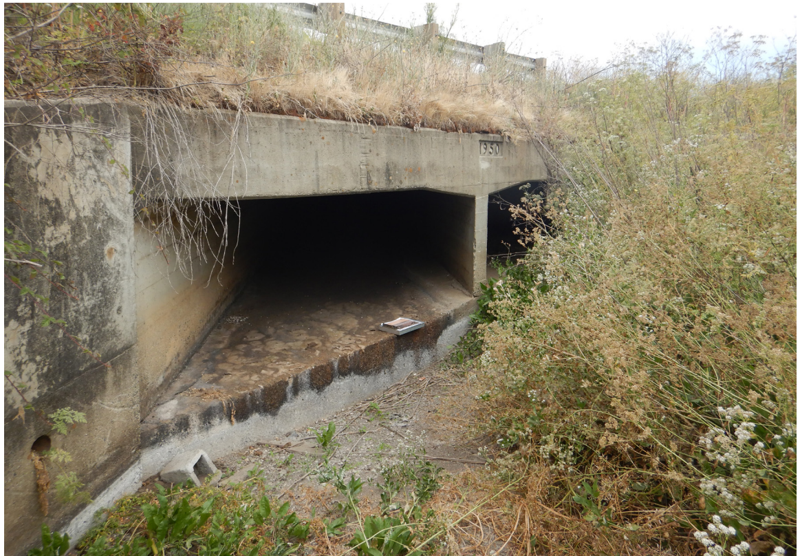
US 101 Site 3 Tick Creek culvert. Photo faces northwest towards the culvert entrance on the northbound side of US 101.
