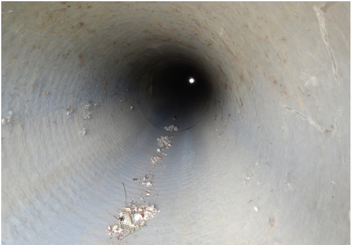
SR 152 Site 6 Tree round culvert. Photo taken from culvert entrance on SR 152 westbound side.
