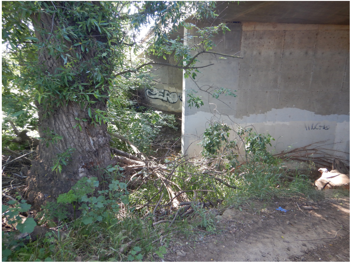
SR 25 Site 1 Carnadero Creek Bridge. Photo from west bank facing southeast towards the east bank.
