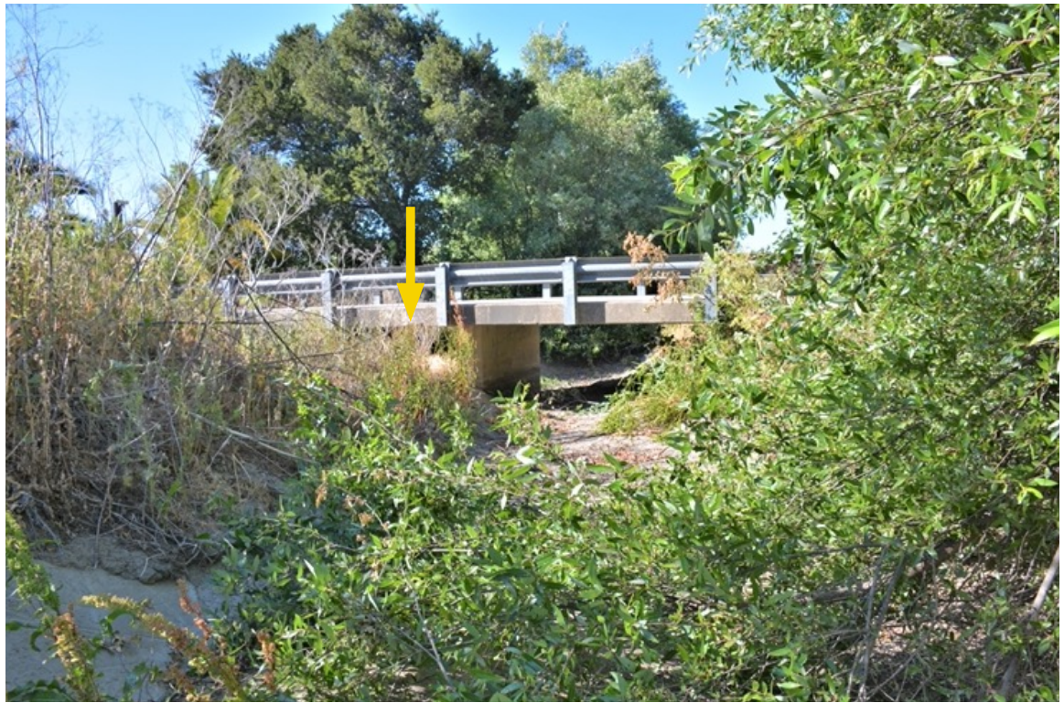
SR 156 Site 6. View of bridge to the north. The levee (indicated by yellow arrow) runs through the western section below the bridge.
