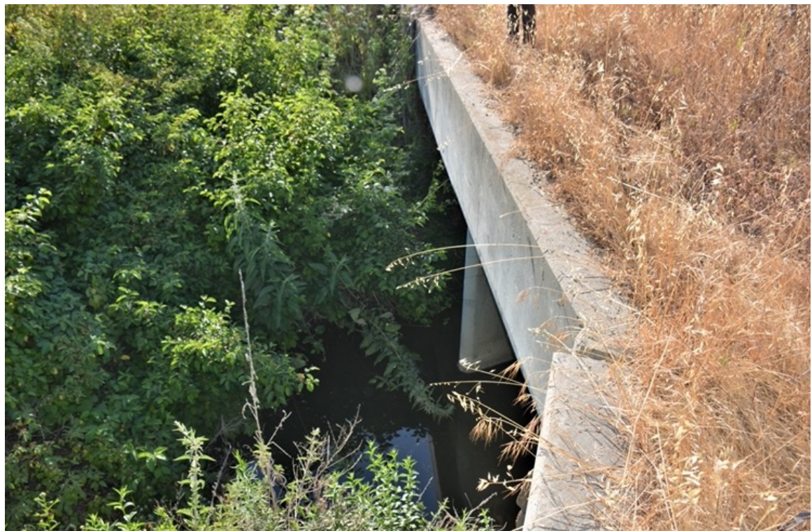
US 101 Site 2. Northern section showing sediment build-up at the northwestern opening.
