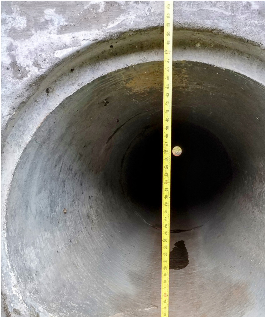
SR 152 Site 4 Coyote and Badger culvert. Photo taken from culvert entrance on SR 152 westbound side.
