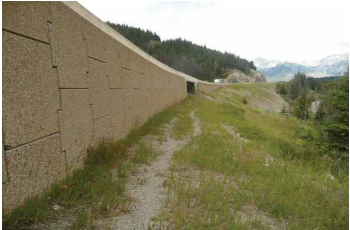
Mechanically stabilized earth wall serving as wildlife exclusion “fence.” Photo by Tony Clevenger.
