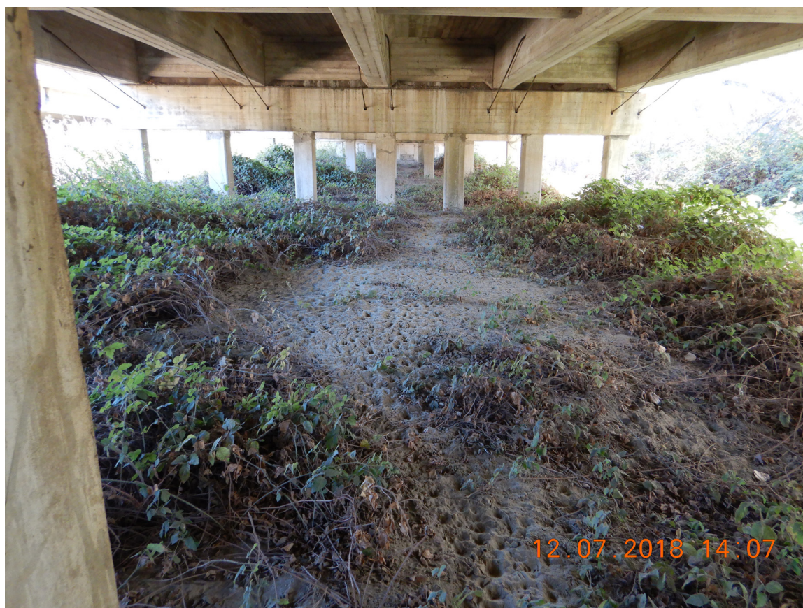
US 101 Site 6 San Benito River Bridge. Photo faces south from north side of San Benito River under US 101 southbound.
