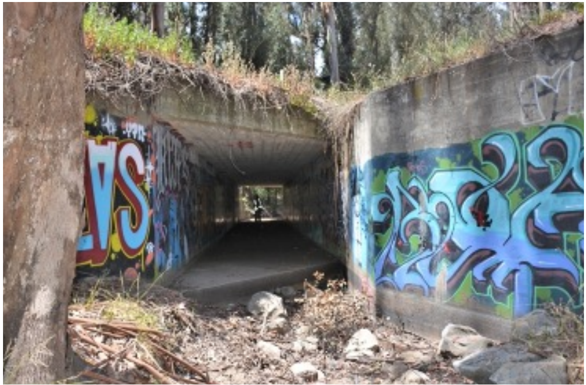
US 101 Site 10. Northern opening with 5' 7" tall person standing near southern opening for scale.
