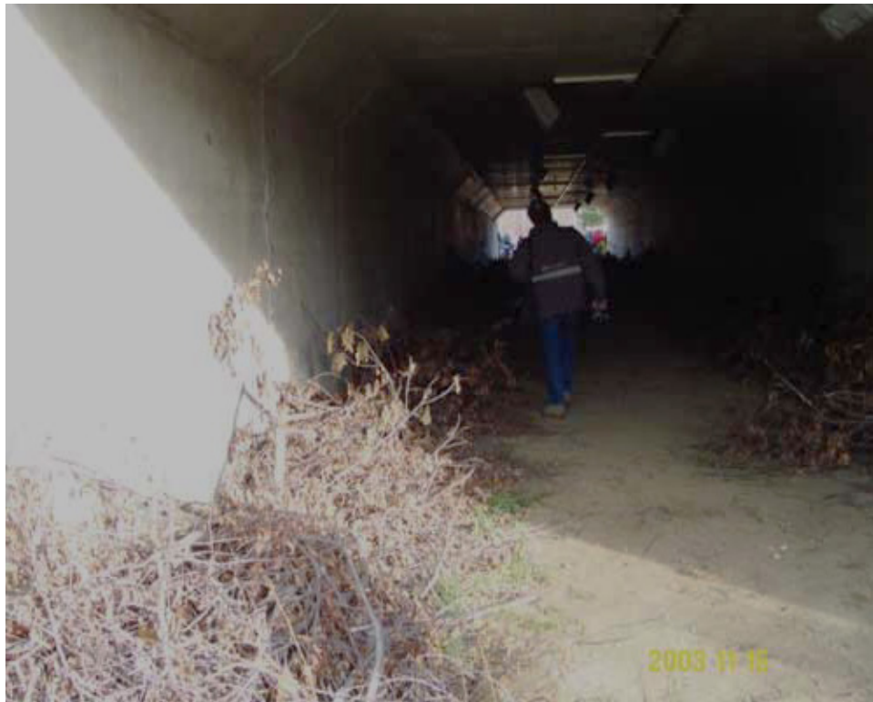
Brush and root wads along the edges of the undercrossing wall provide cover for mammals Photo by Nancy Newhouse.
