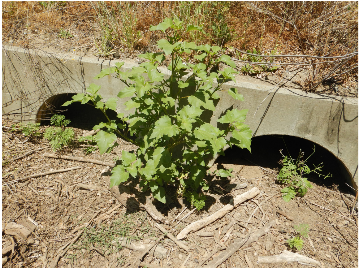
SR 152 Site 1 San Felipe Lake dual round culverts. Photo faces northwest towards culvert entrance on SR 152 eastbound side.
