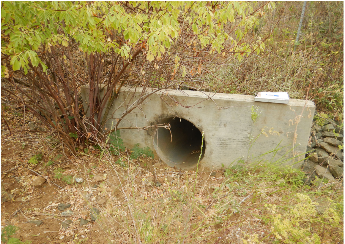
SR 152 Site 6 Tree round culvert. Photo of culvert entrance on SR 152 westbound side.
