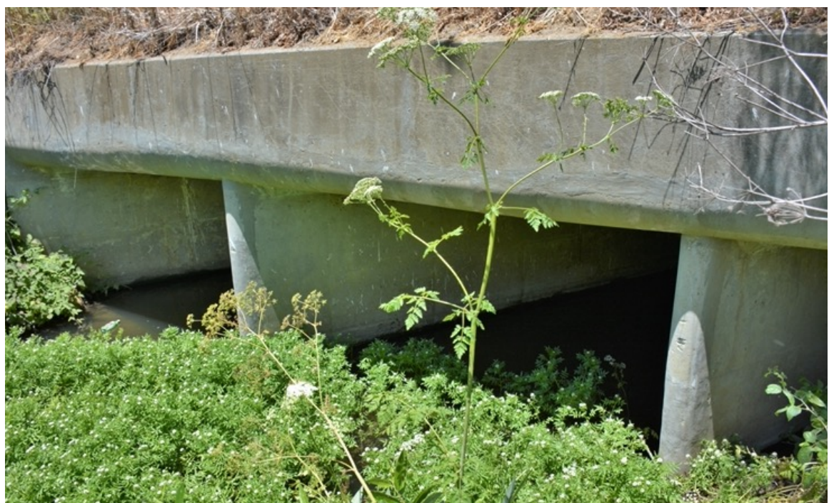
US 101 Site 1. Southeastern opening showing the three sections of the culvert—from left to right, southern, center, and northern sections. Photo faces west.
