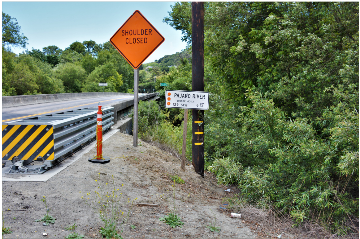
SR 129 Site 5 Pajaro River Bridge. Postmile marker of Pajaro River Bridge and SR 129. Photo faces east.
