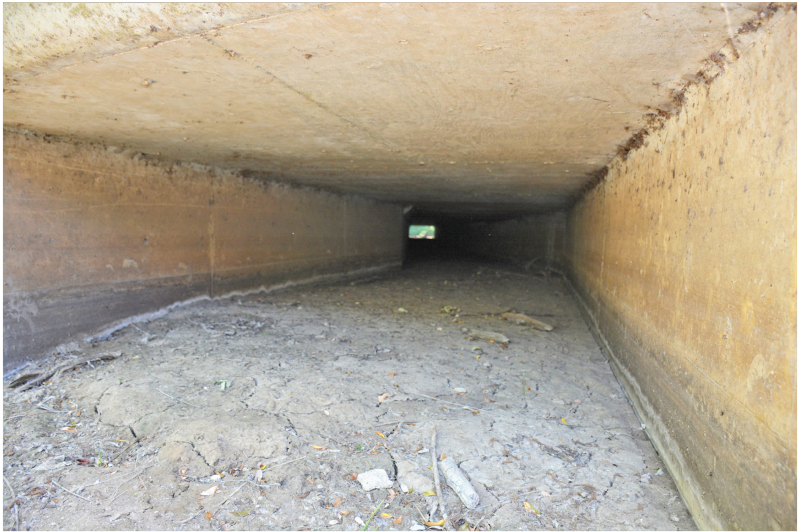
SR 156 Site 6. View from within northern opening of western culvert. The eastern bend toward the southern opening is visible. Photo faces south
