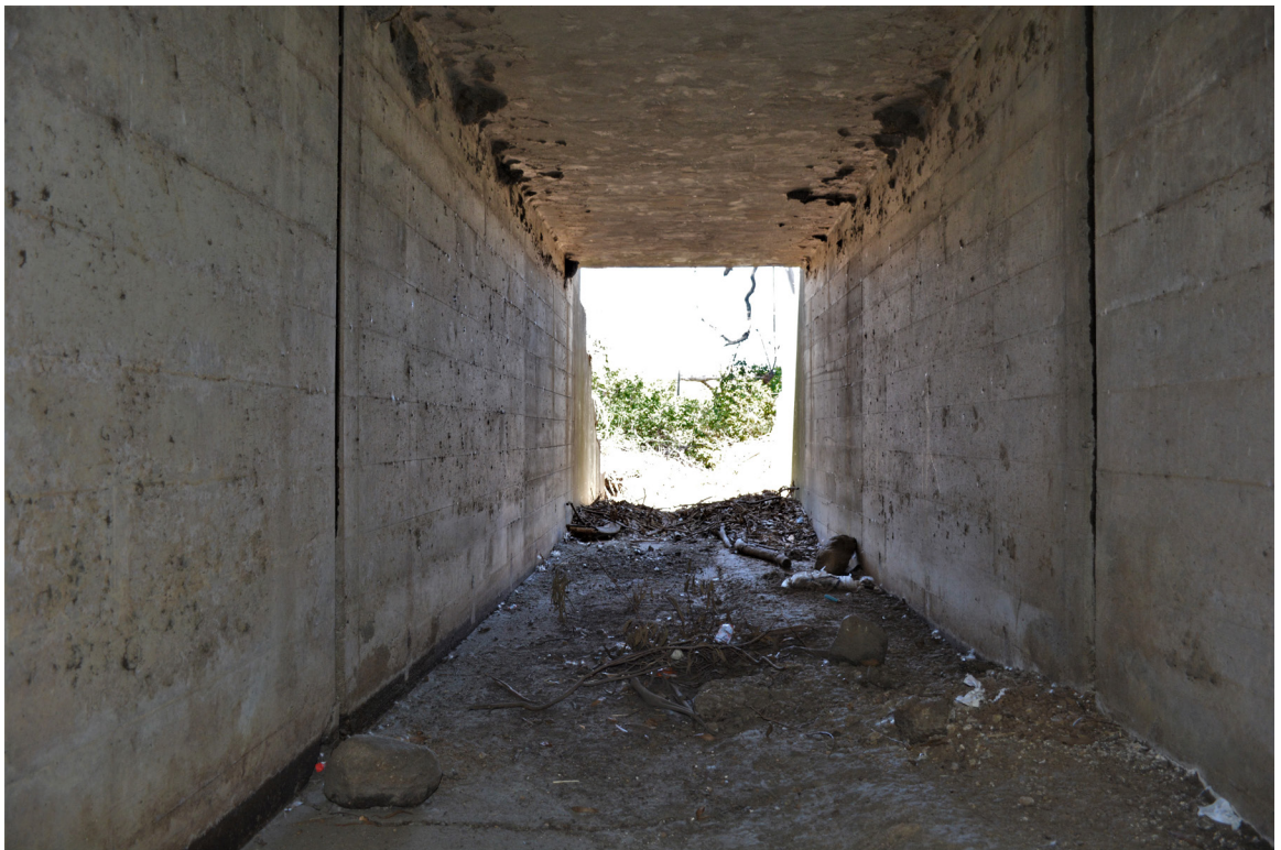
SR 156 Site 1. Photo from within the culvert faces outward from the northeast opening.
