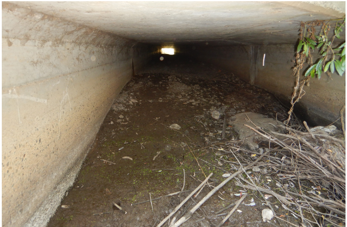
US 101 Site 3 Tick Creek culvert. Photo from the southbound side of US 101 faces southeast through the northern box.
