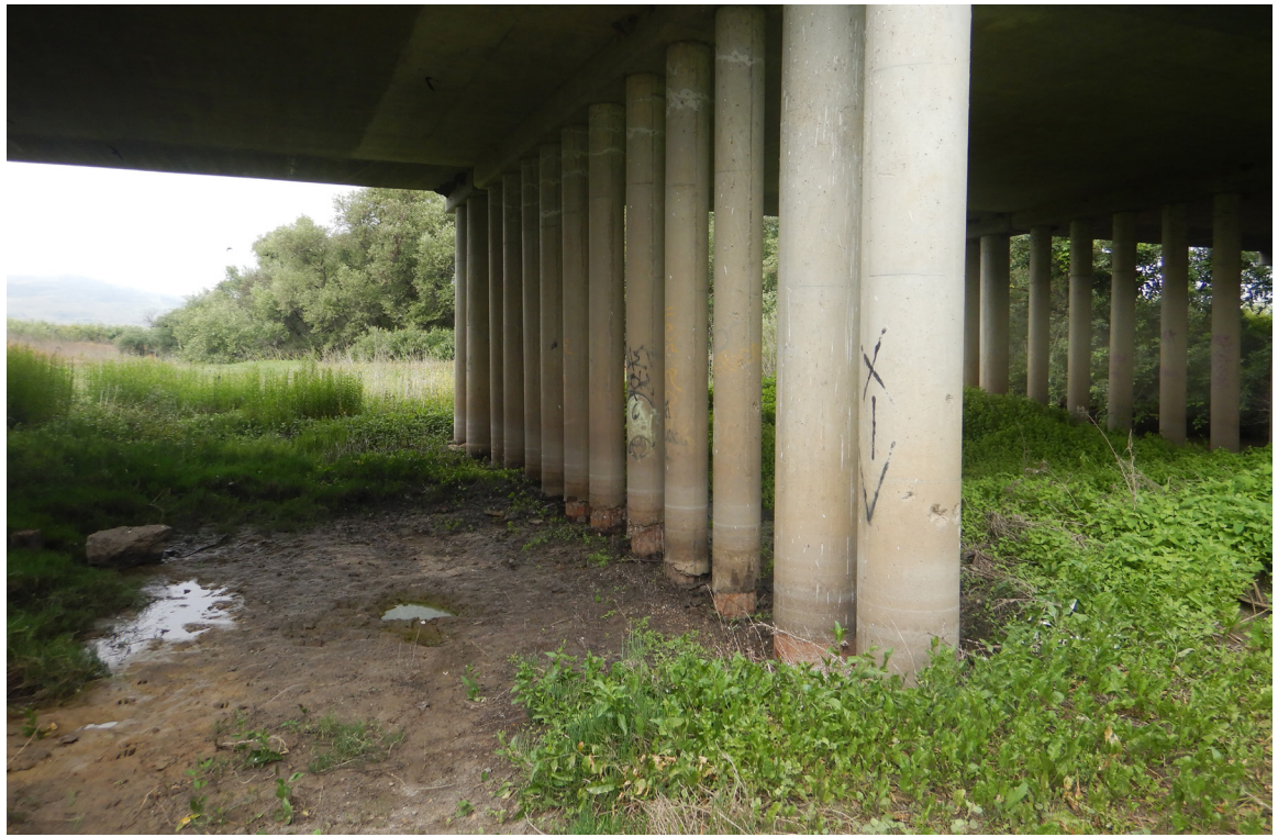
SR 25 Site 2 Pajaro River Bridge. Photo faces northeast along the west bank.
