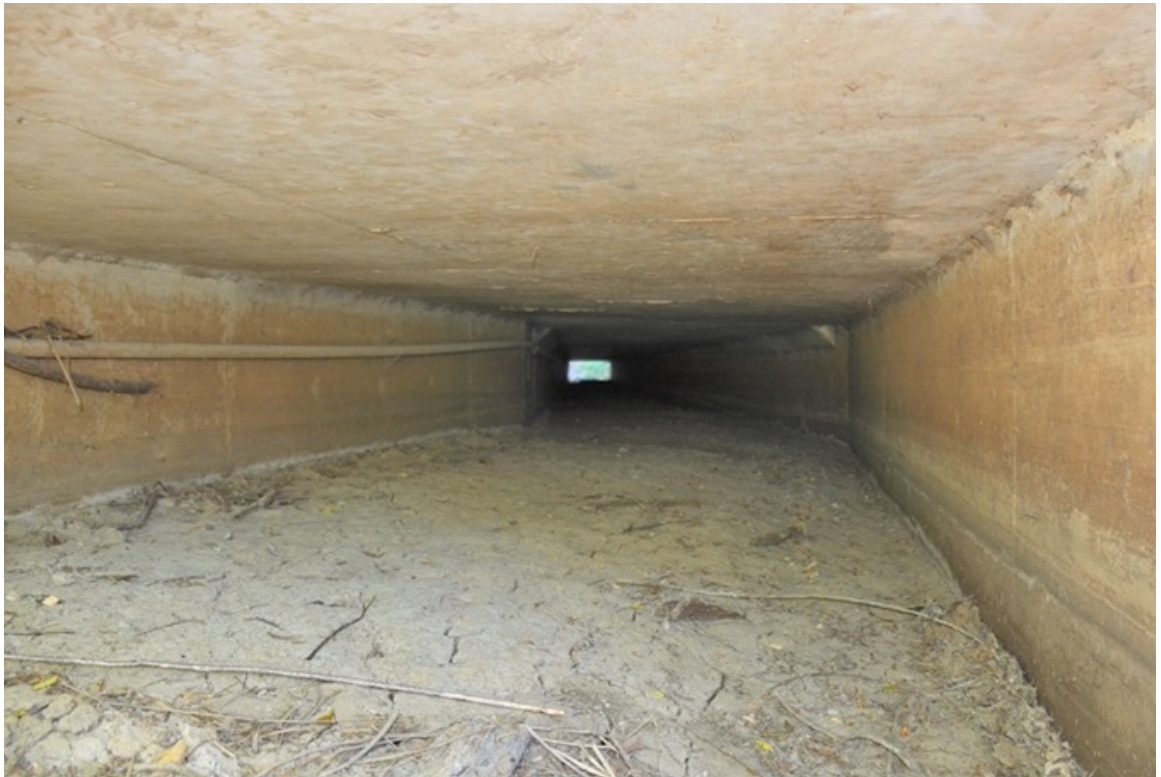
SR 156 Site 6. View from within northern opening of eastern culvert. Eastern bend in culvert identical to western culvert. Photo faces south.
