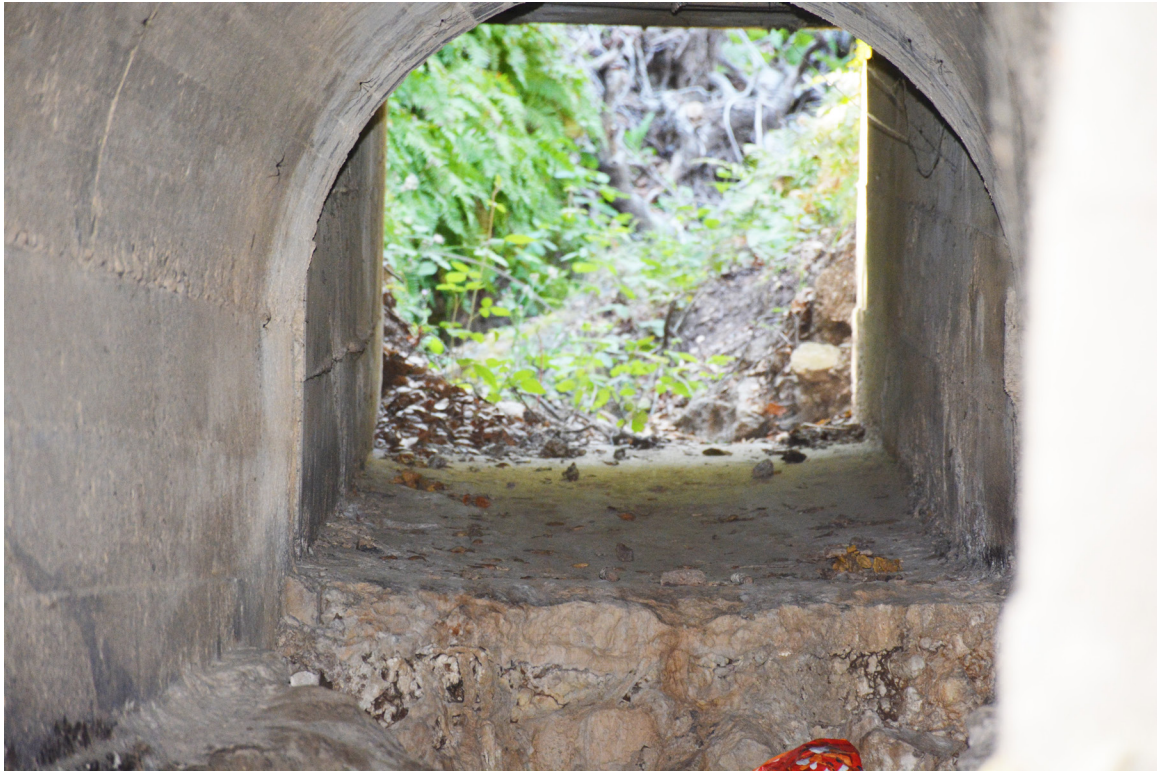
SR 129 Site 8. Photo shows drop in midway through the culvert. Photo faces northwest.
