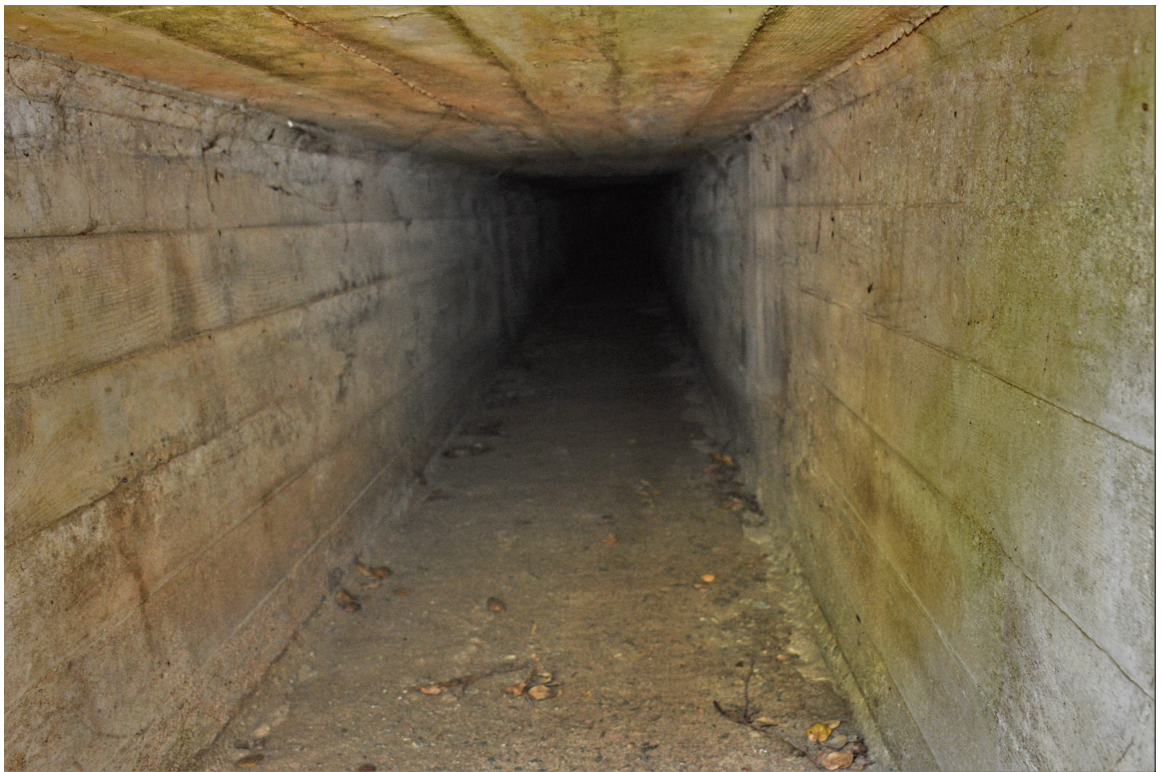
SR 129 Site 3. Within southwest opening of culvert. Photo faces northeast. The northeast end of the culvert is not visible.
