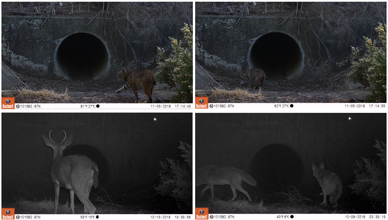
Wildlife approaching but not traveling through the culvert at US 101 Site 7. This culvert is angled and obscured by brush, and visibility is poor.
