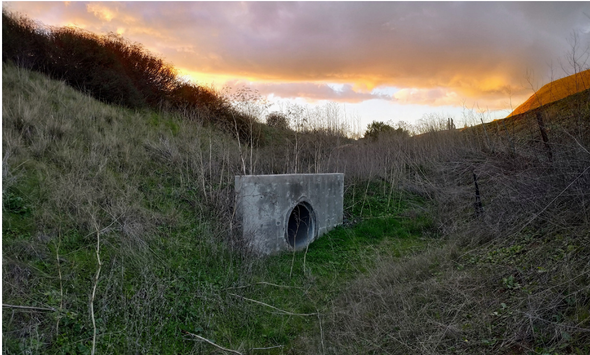
SR 152 Site 4 Coyote and Badger culvert. Photo of culvert entrance on SR 152 westbound side.
