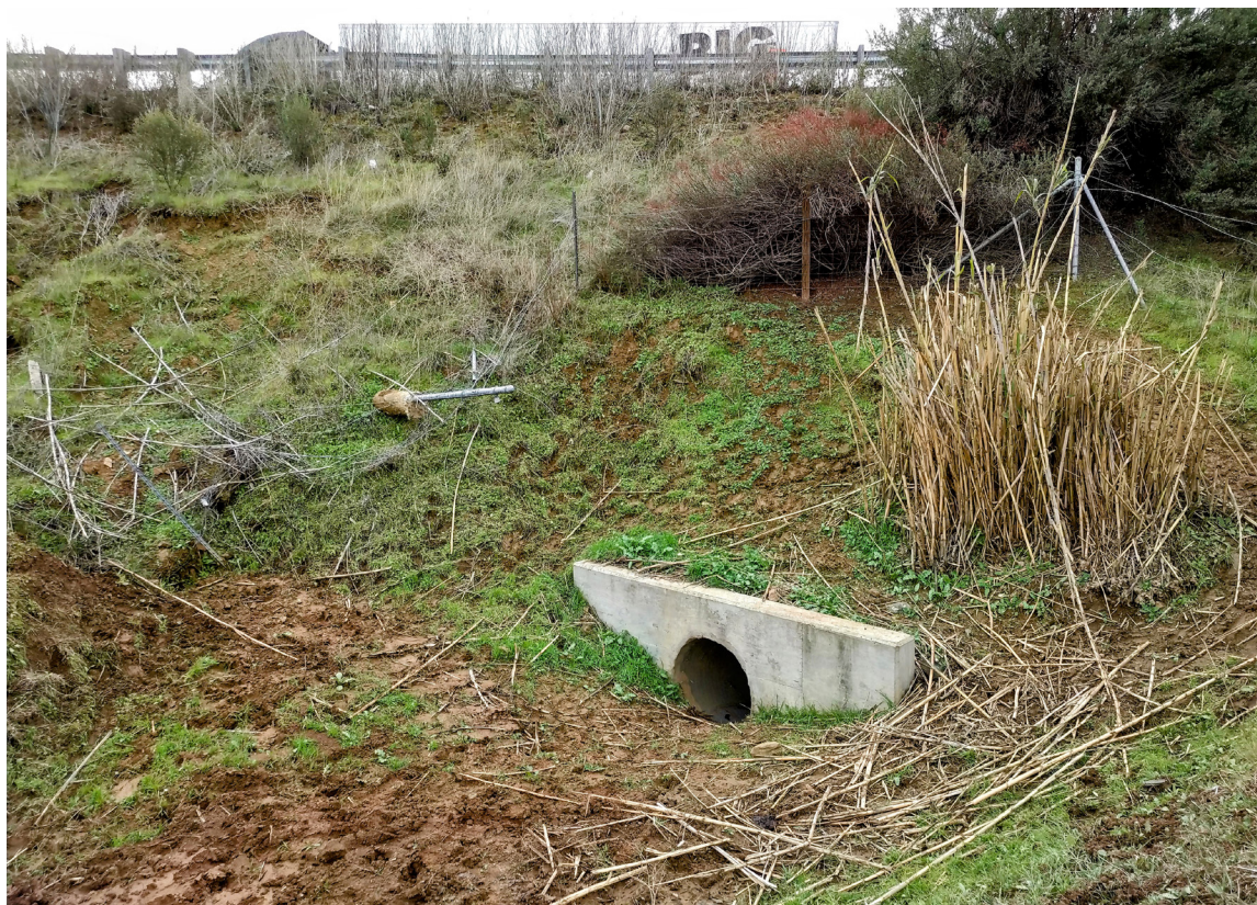
SR 152 Site 5 Coyote Puppy culvert. Photo of entrance on SR 152 westbound side.
