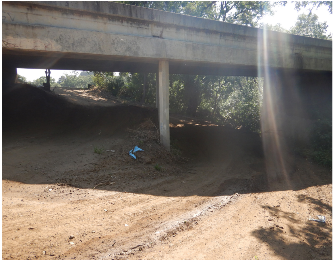
SR 25 Site 1 Carnadero Creek Bridge. Photo faces northeast along the west bank.
