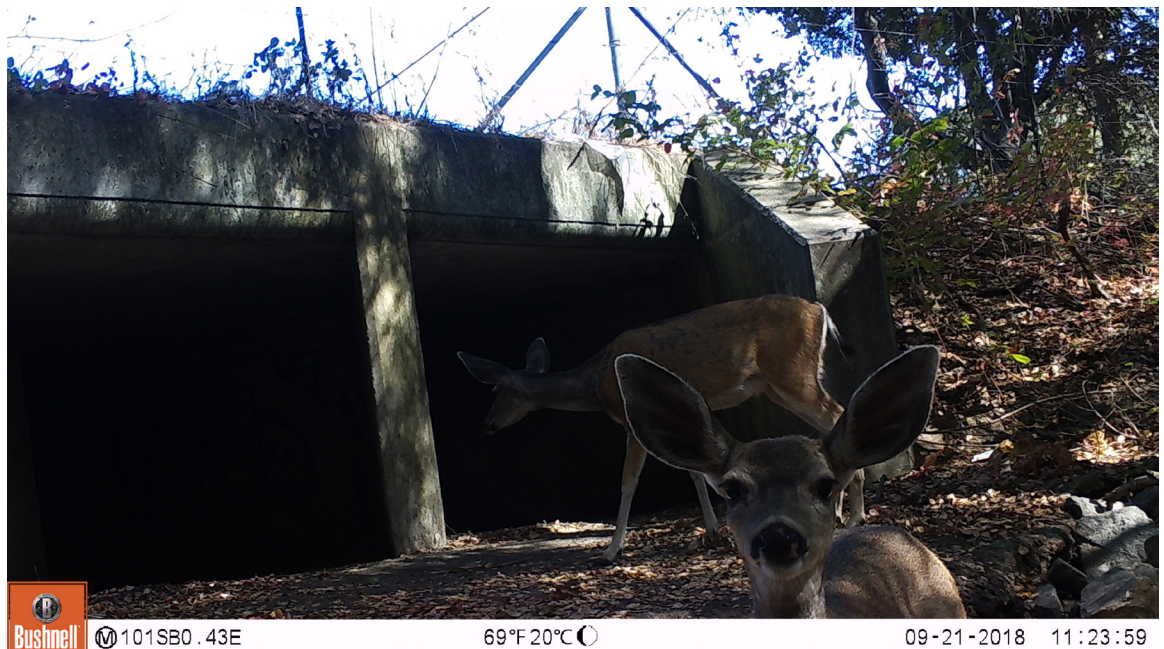
Deer approaching but not traveling through the pair of box culverts at US 101 Site 17.
