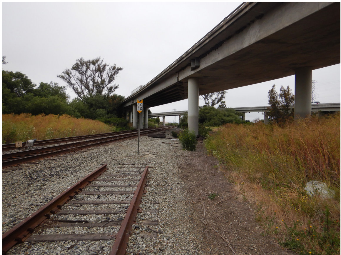
US 101 Site 4 Tar Creek Overpass. Photo faces east from west side of US 101 southbound.
