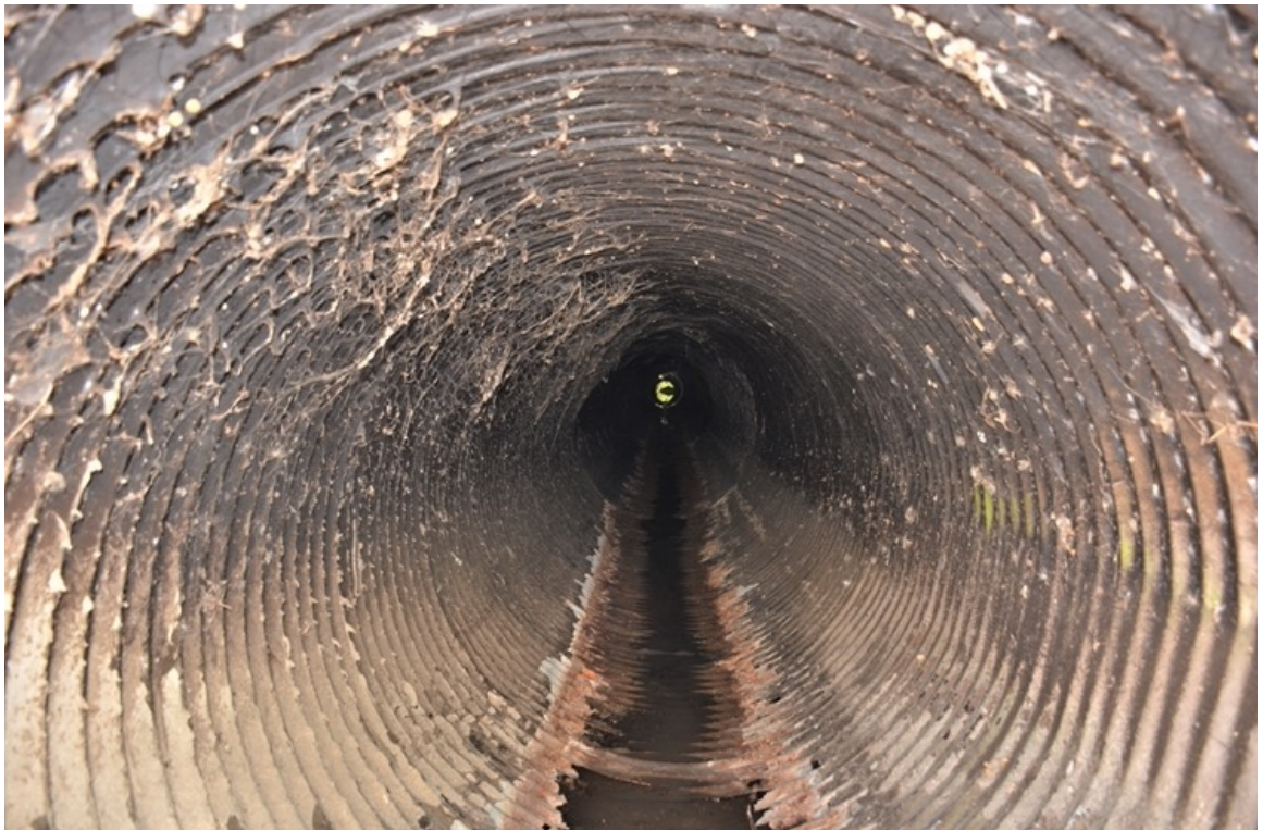
US 101 Site 5. Within northwestern opening, showing the corroded bottom of the culvert.
