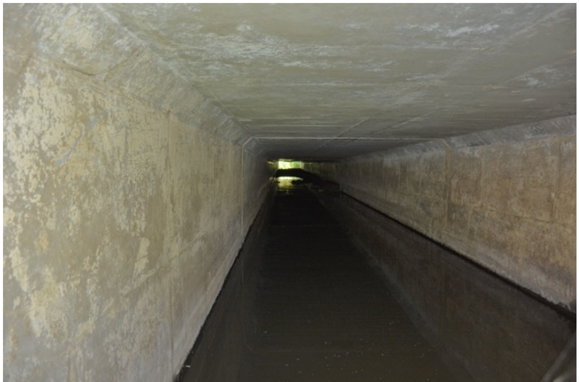
US 101 Site 1. View of northern section showing sediment build-up at the northwestern opening.
