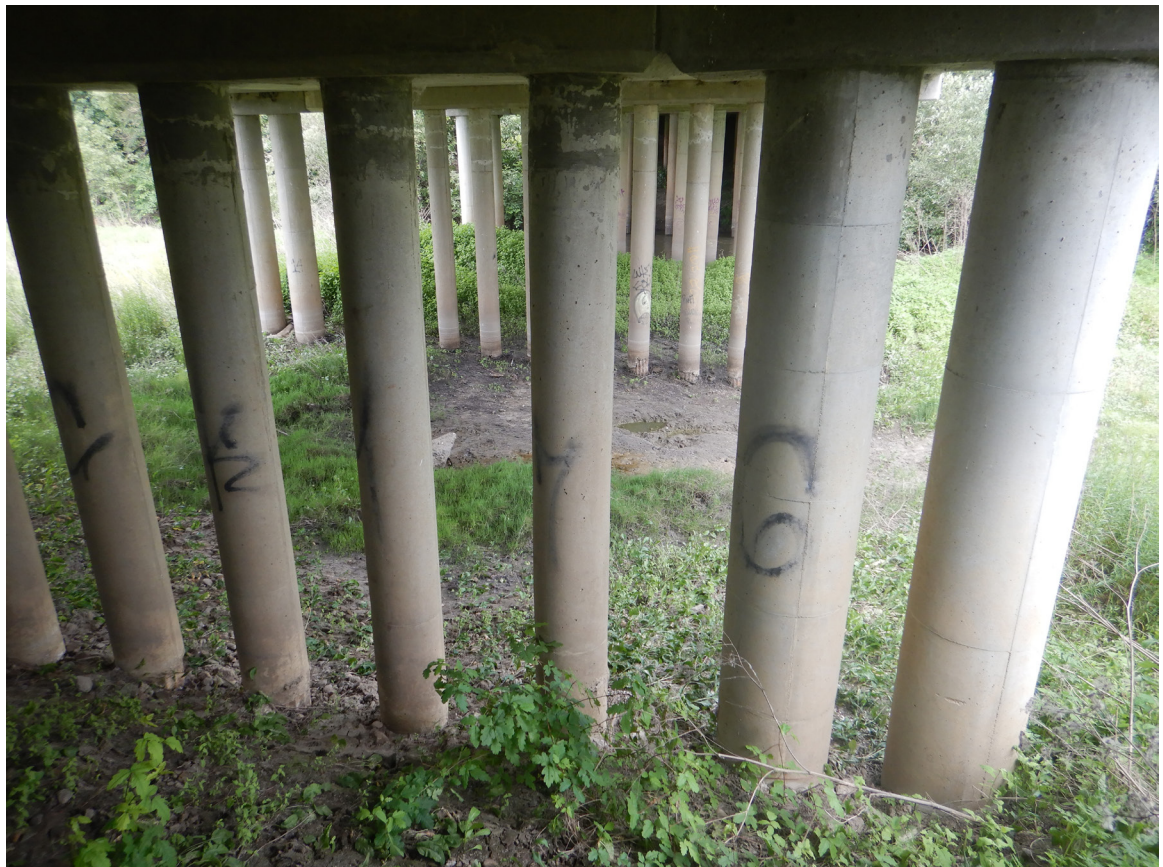
SR 25 Site 2 Pajaro River Bridge. Photo from west bank faces southeast towards the east bank.
