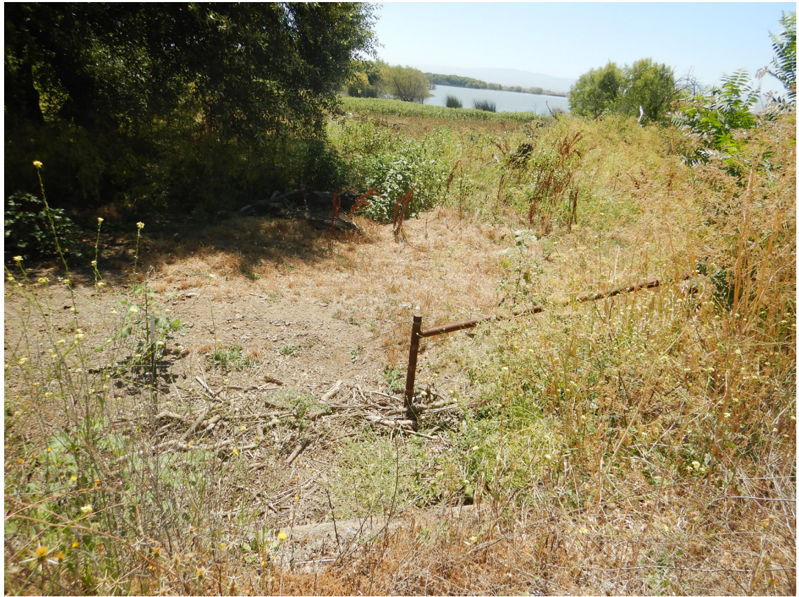
SR 152 Site 1 San Felipe Lake dual round culverts. Photo faces southeast away from the culvert entrance on the SR 152 eastbound side.
